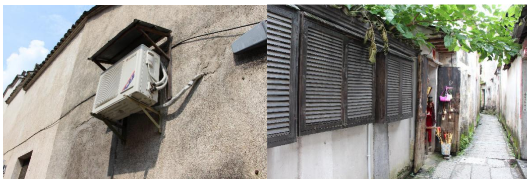
Figure 2-1 Air conditioning exhaust fans
