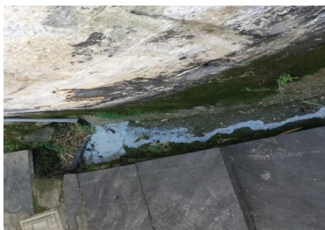
Figure 7-4. sewage in the channel
